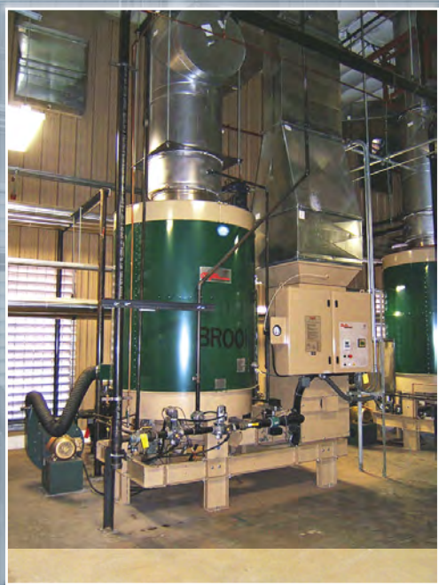
Whether it's new construction or a retrofit, owners appreciate the small footprint of a coil tube boiler, as with this Clayton compact vertical unit in a grain processing plant. Photo courtesy Clayton International.
