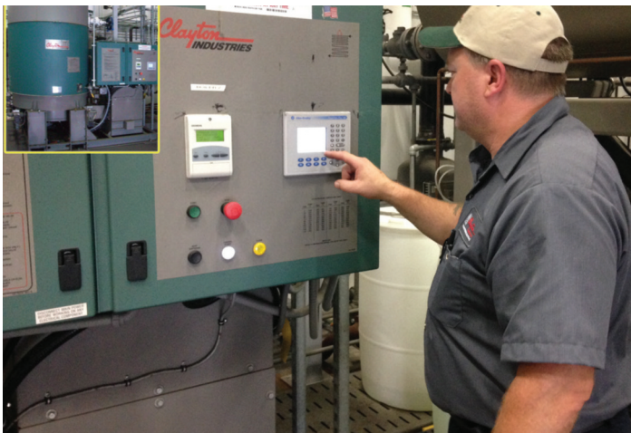
▶ Kettle Cuisine installed Clayton Industries Model SE254 steam generators with economizers at its Lynn, MA, facility. Each generator provides 8,625 pounds of steam per hour. Source: Clayton Industries.
