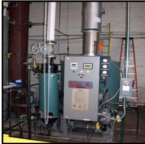
Clayton Steam Generator
