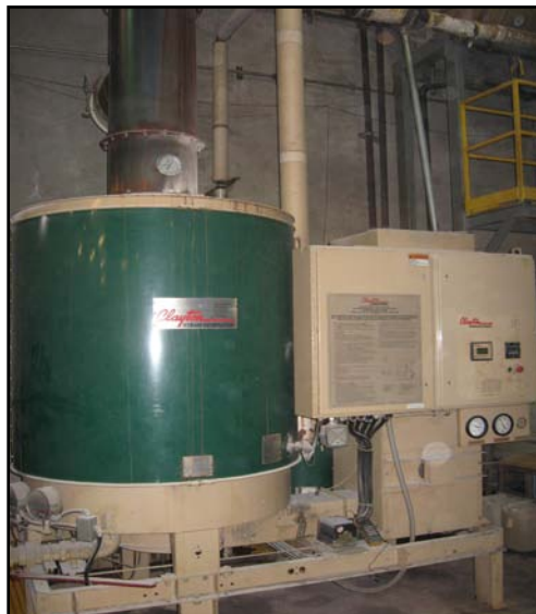
Clayton Steam Generator at Jost Chemical
