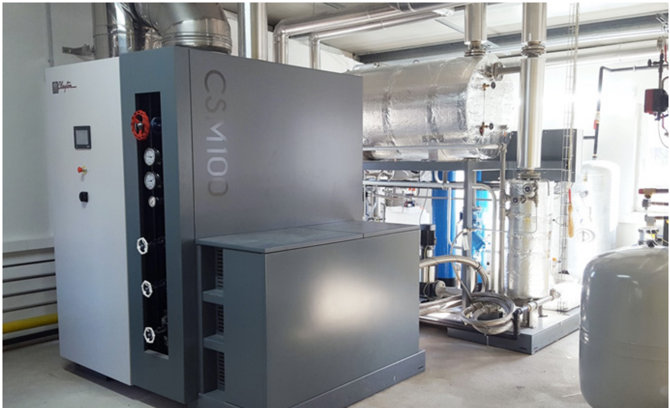
The Steam Master CSM100 shortly after its commissioning in Fürnitz.
