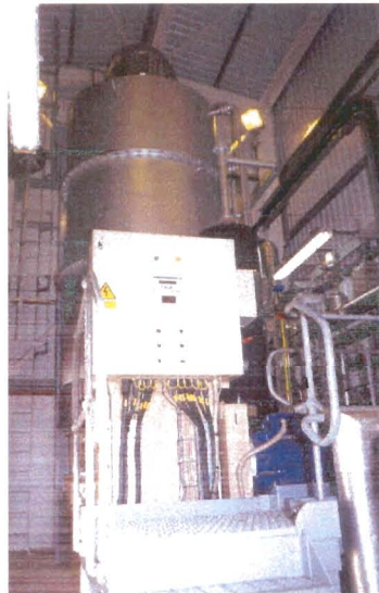
The Clayton Steam Generator
