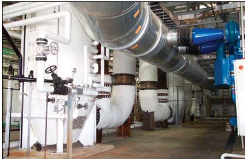
Exhaust gas boilers (the tall, white vertical equipment on the left) are heated by the waste heat stream from the process rather than from their own burner. In this installation, the metal duct in the top center of the photo is the air intake for the natural gas internal combustion engines. The intake duct connects to the blue duct on each engine.
