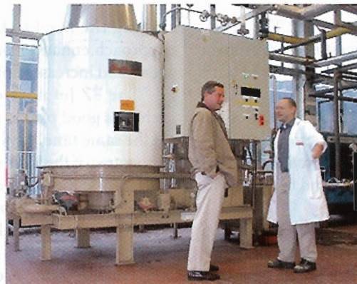
After installing an immense new autoclave to its Puurs facility, Campbell Foods purchased a large steam generator that maintains a constant supply of steam to all kettles and autoclaves. Source: Campbell Foods Belgium.
