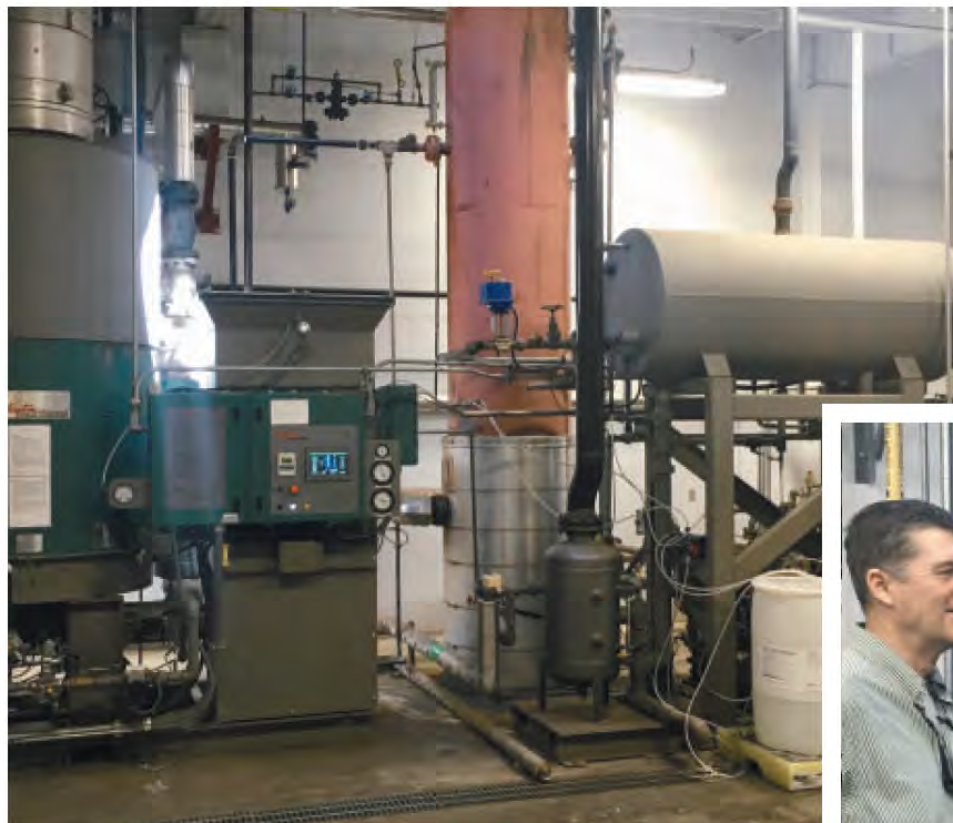
Clayton steam generator installed at a Pacific Southwest Container facility.
