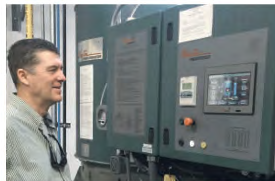
Clayton's Chip Maguire checks the readout on the steam generator.
