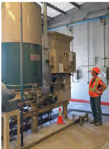
Bronco Wine Company Maintenance Supervisor Jason Paillor checking operations of a Clayton Steam Generator in Escalon, Calif. Photo courtesy Bronco Wine Co.
