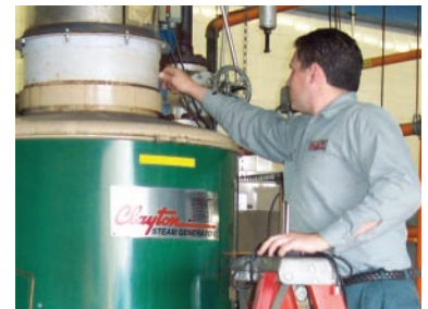
On Location – Knowledgeable and experienced Clayton professionals solve steam generation problems at your plant.
